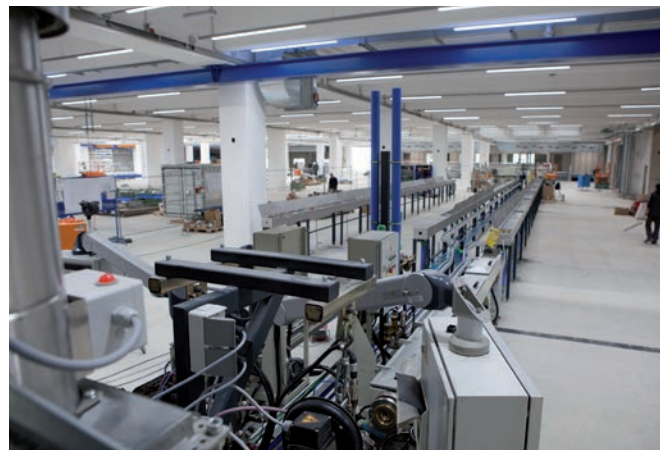
Week 32 Trial operation of the first plant in ZuRo
