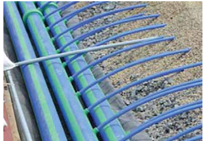
The supply and return lines along the edge of the field, with the fusion outlet-connected coil tubing covered by sand.
