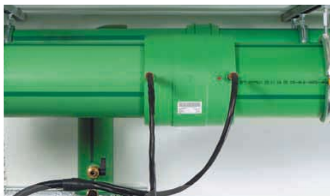
Adjust the socket diameter on the welding device. Start and control welding process. Keep the cooling time. Finished!
