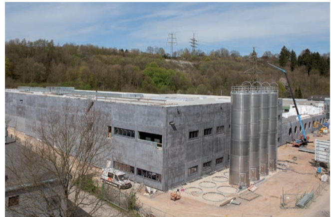
View from the administration building: Here, later on 12 silos will be placed for the supply with raw material
