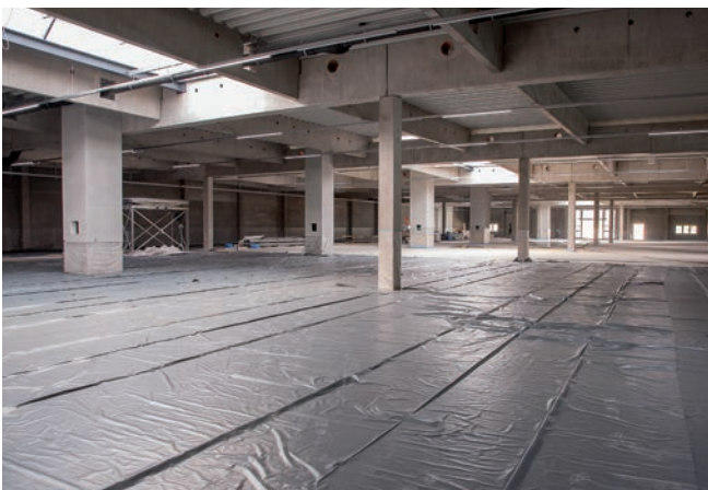
On the upper floor, the periphery for raw material supply is formed
